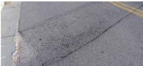
Top: T-Lock repair without the GlasGrid System Right: T-Lock repair with the GlasGrid System
