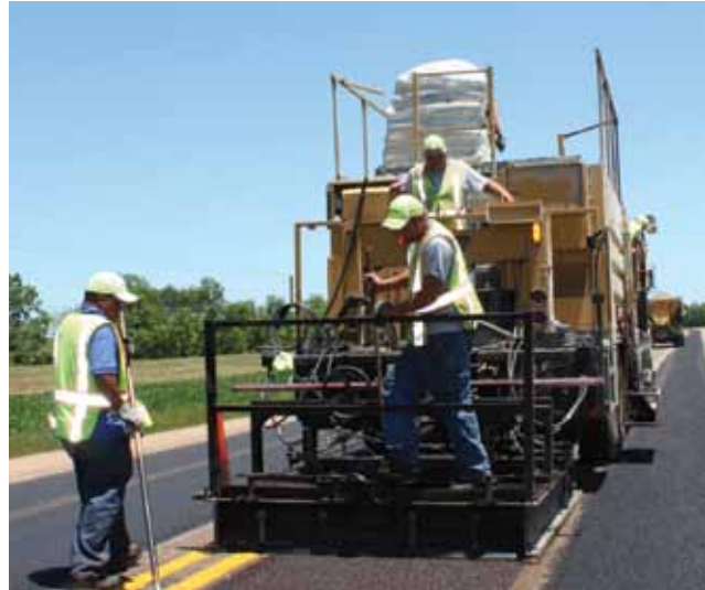
A feeder truck (above) supplies densely graded sandstone to the asphalt emulsion treatment being applied in a single pass with the Bergkamp paver (below).
